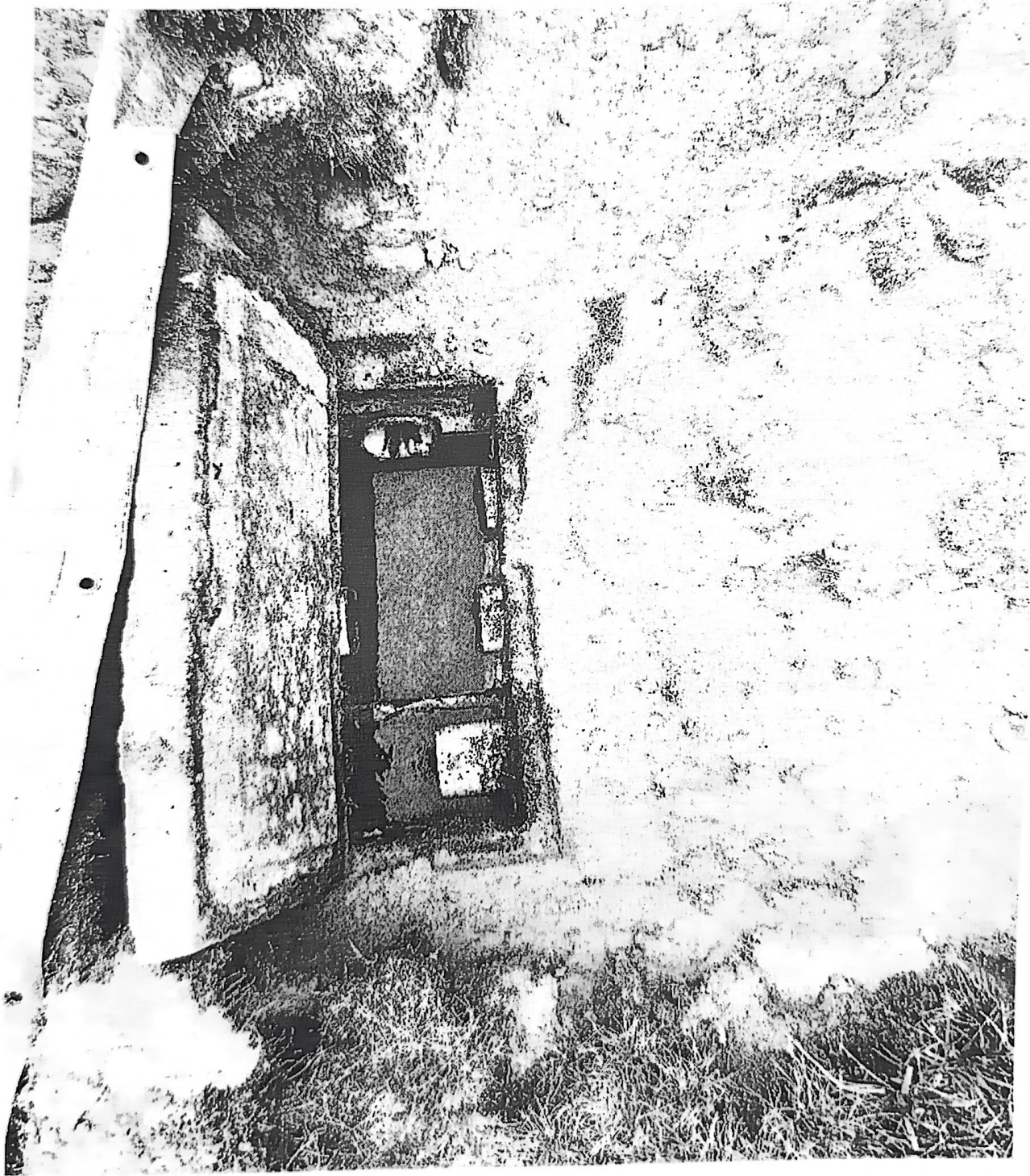
5 Outlet distribution box 4 outlets used on system.
