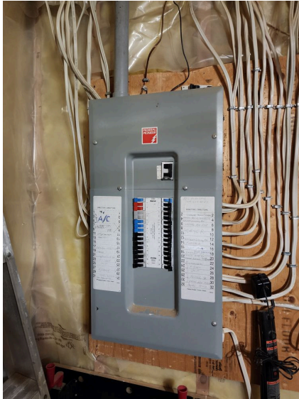
Main electrical disconnect
