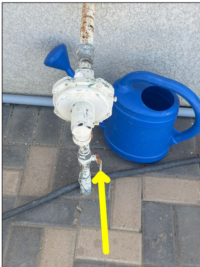
Main gas shut off to the home.
