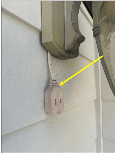
Extension cord used as permanent wiring was visible at the front of the garage.
