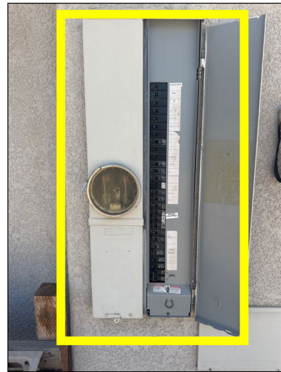
Main electrical service panel to the home.
