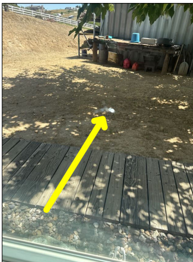
A window had a cracked or broken pane.
