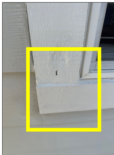
Moisture damage, wood rot, observed.
