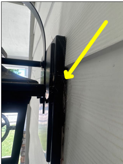
Exterior lighting was loose/not flush to the wall and could expose electrical components to moisture intrusion. front door
