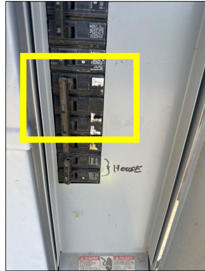
Main electrical shut off to the property
