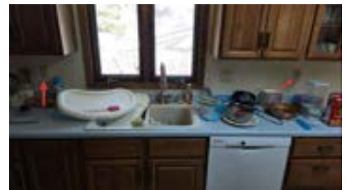
1st Floor Kitchen Outlets No GFCI Protections
