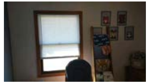
1st Floor Back Bedroom Window Wont Stay Open
