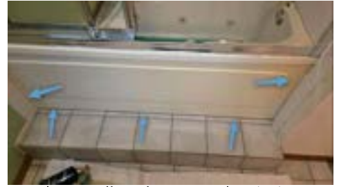
1st Floor Hall Bathroom Tub Missing Caulking
