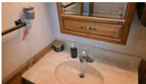
Basement Hall Bathroom Outlet No GFCI Protection
