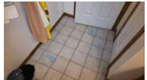
1st Floor Hall Bathroom Cracked Tile
