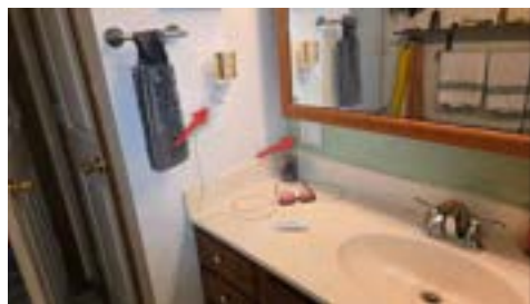
1st Floor Hall Bathroom Outlets No GFCI Protections
