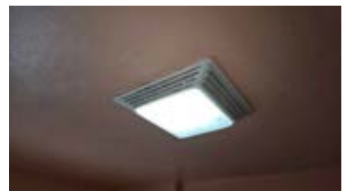
1st Floor Hall Bathroom Vent
