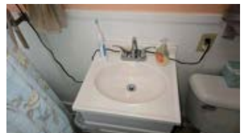
1st Floor Hall Bathroom Sink Cold Water Significantly Lower Water Pressure Compared To Hot Water
