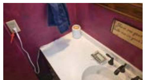
1st Floor Bathroom Outlet No GFCI Protection
