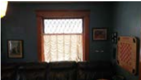
1st Floor Livingroom Window Damaged and Missing Balances
