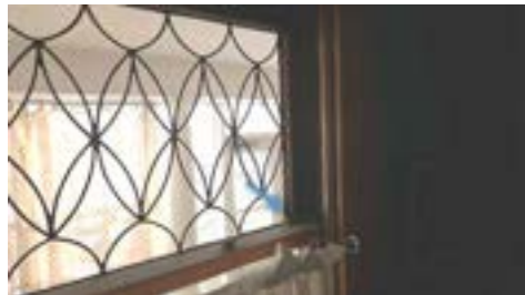
1st Floor Livingroom Window Damaged Balances
