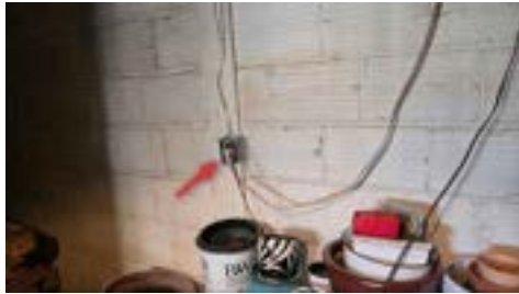
Basement Room Outlet
