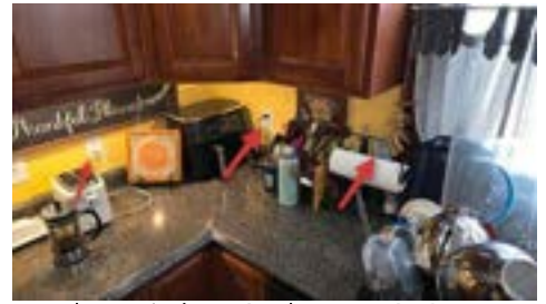
1st Floor Kitchen Outlets No GFCI Protections
