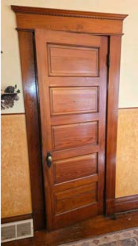
1st Floor Dining Room To Hall Door Can't Latch
