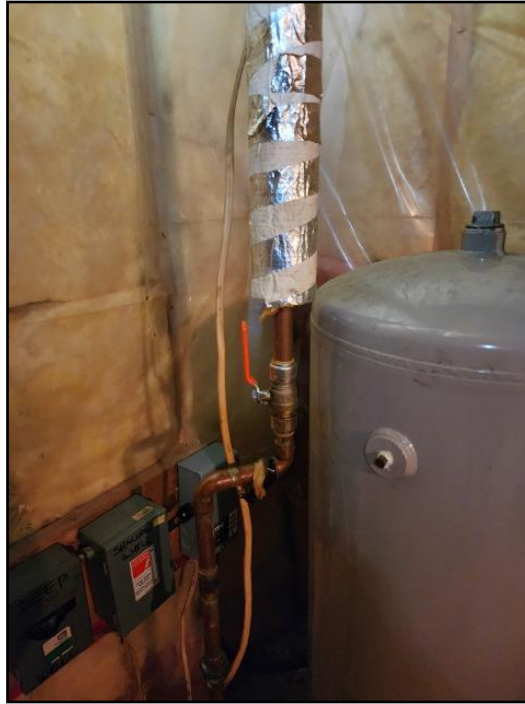
27. Main water shut off
