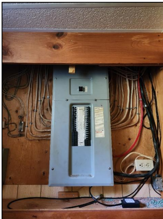
5. Main electrical disconnect
