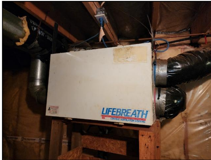
18. Heat recovery ventilator (HRV)
