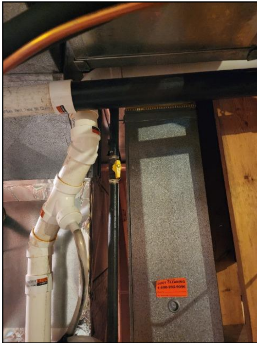
12. Main fuel shut off
