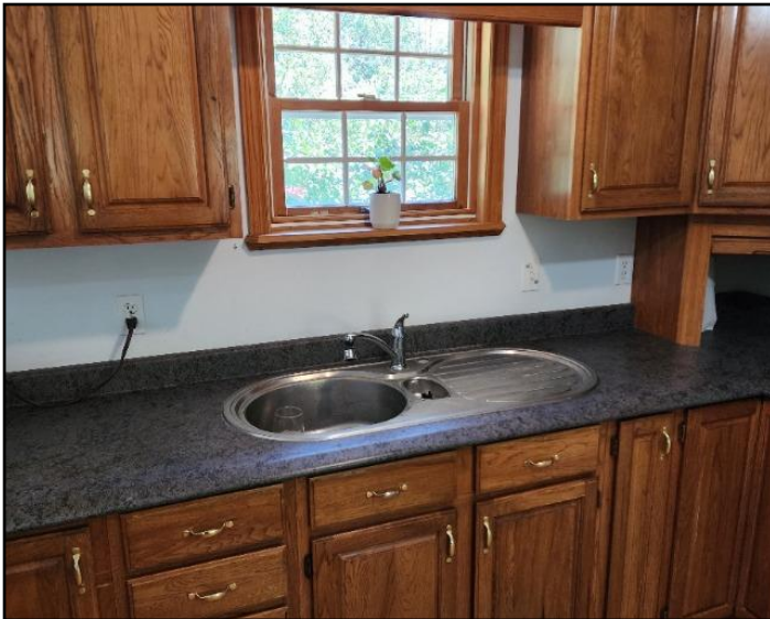
7. No GFCI/GFI (Ground Fault Circuit...
