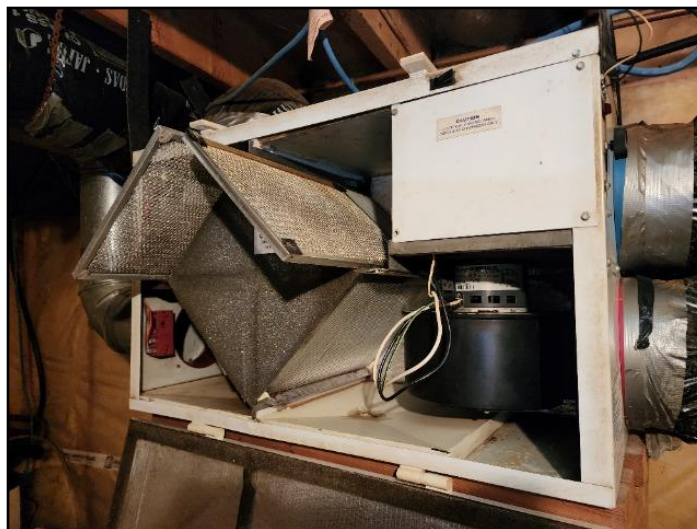
22. Clean filters - regular maintenance
