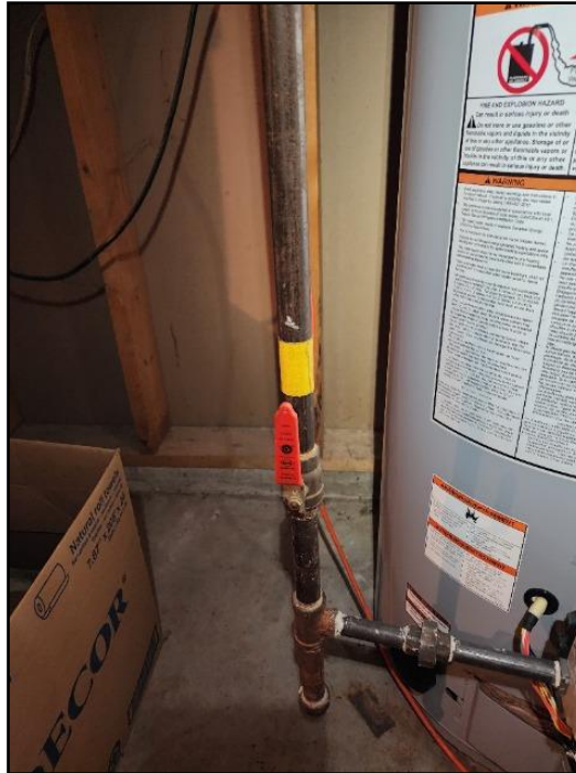
32. Main fuel shut off
