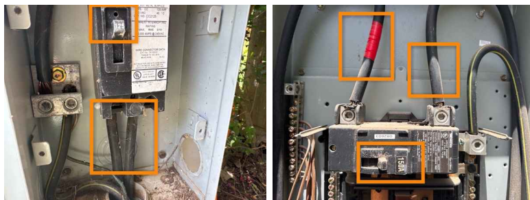
Main service panel in the backyard
