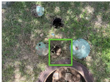
Main water shut off valve
