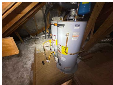
View of the water heaters in the attic
