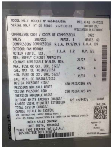
Data plate information for the downstairs exterior AC unit
