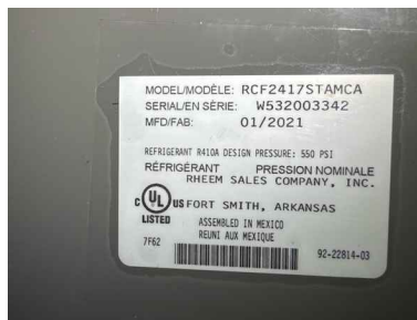
Data plate information for the upstairs air handler
