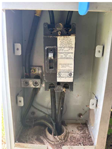
Main service panel in the backyard
