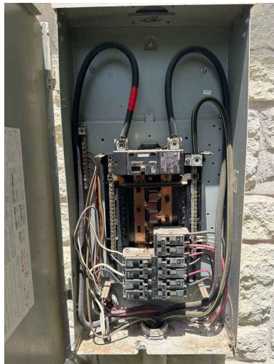
Exterior electrical panel at the left side of the home
