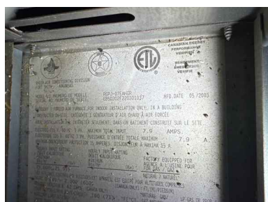
Data plate information for the downstairs furnace
