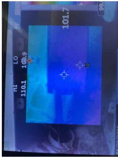
Thermal limit of the main service panel in the backyard
