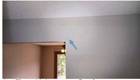
1st Floor Livingroom Crack
