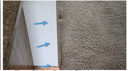
1st Floor Dining Room Crack
