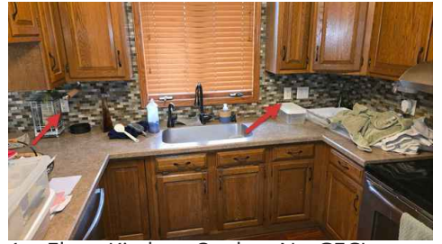
1st Floor Kitchen Outlets No GFCI Protections
