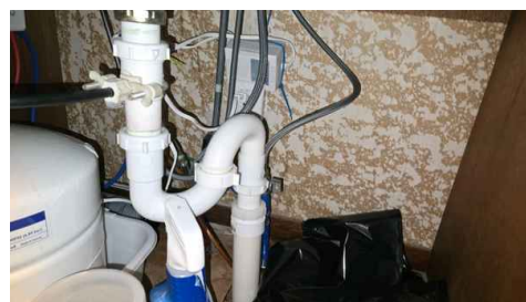
1st Floor Kitchen Sink
