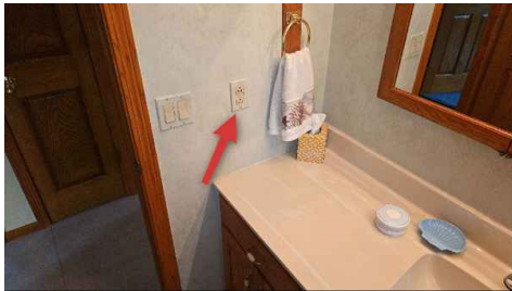
1st Floor Hall Bathroom Bathroom Outlet Improperly Wired and Loose
