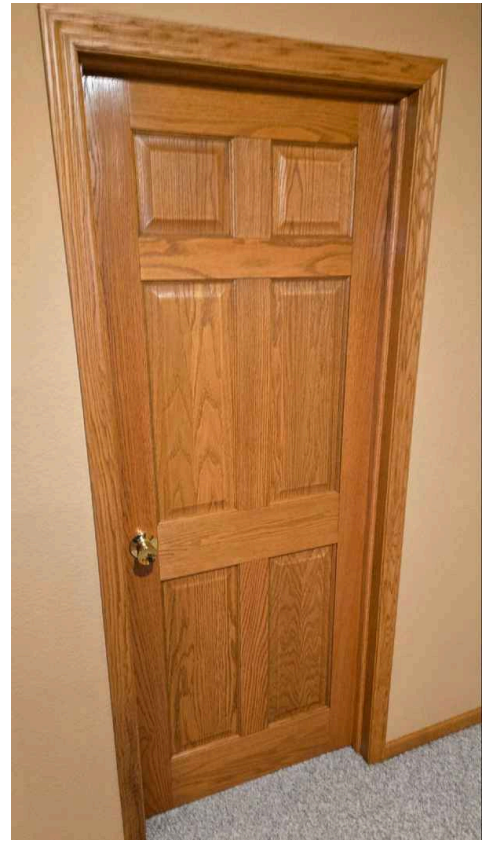
Basement Bedroom's Door Wont Latch and Drags on Carpet
