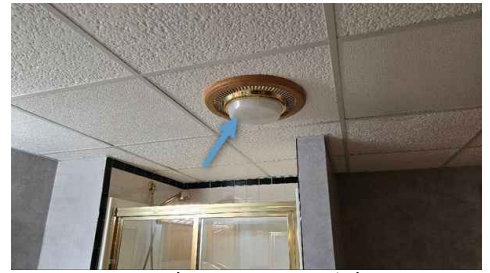
Basement Bathroom Vent Light
