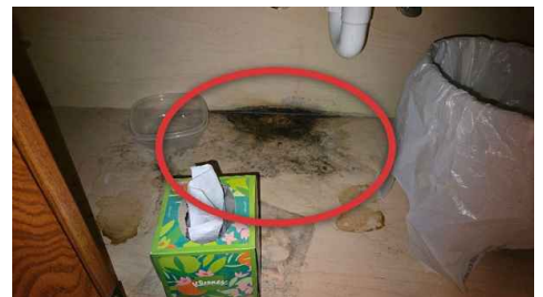
1st Floor Hall Bathroom Sink Inside Cabinet
