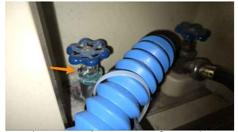
1st Floor Laundry Room Left Supply
