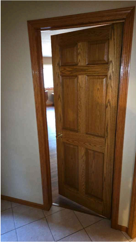
1st Floor Livingroom Door Missing Striker Plate and Wont Latch
