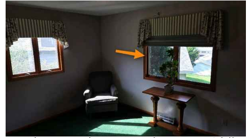
1st Floor South West Bedroom's Middle Right Window (When Trying To Open Gets Sticking On Top)
