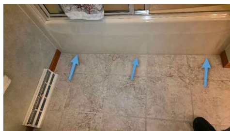
1st Floor Hall Bathroom Tub Missing Caulking
