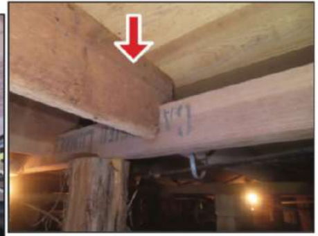
Damage to joist observed
