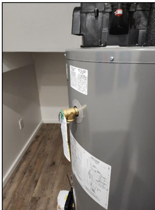
32. Discharge tube missing
