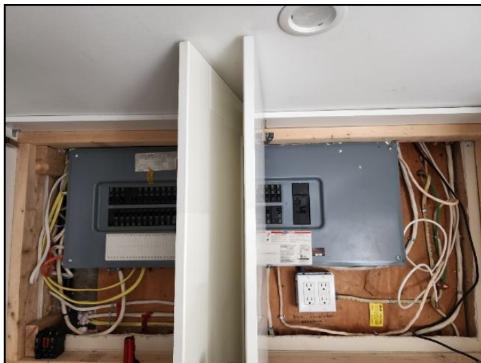
5. Main electrical disconnect
