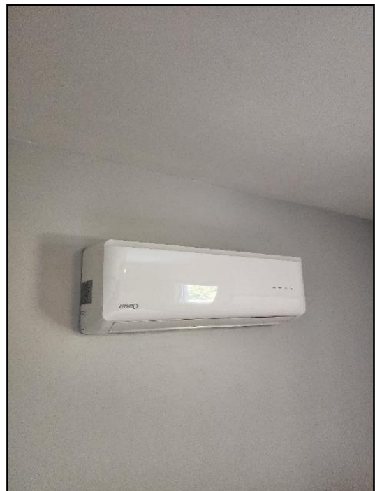
24. Wall mounted heating/cooling units
