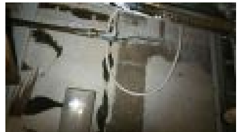
Basement Wet Bar Sink Water Supply Disconnected
