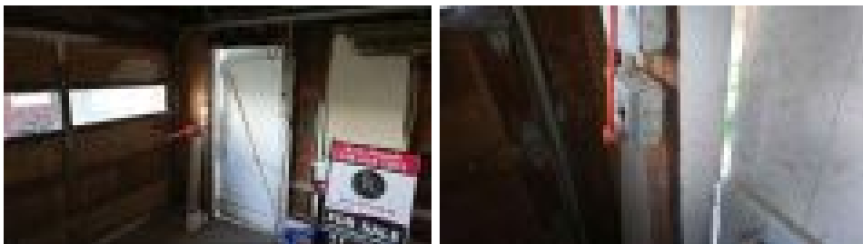
Garage Outlet Loose
