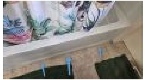
1st Floor Hall Bathroom Tub Missing Caulking
