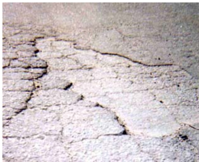
Peeling Thin Pavement Patch
