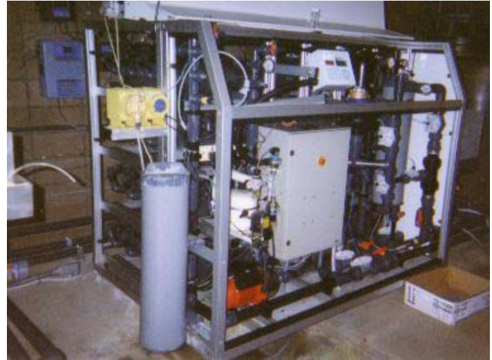
Water Treatment Plant Filtration Equipment
