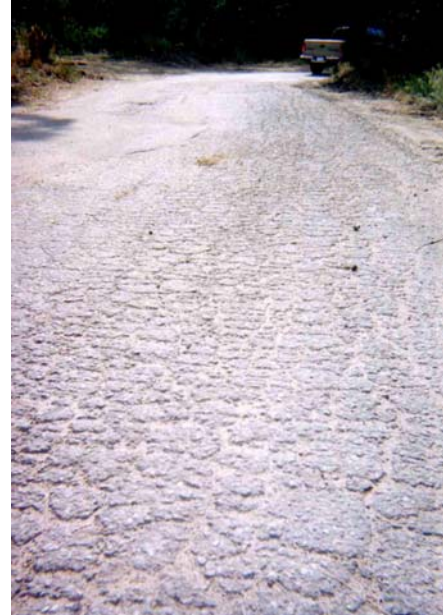
Typical Condition of Access Road Showing Alligator Cracking
