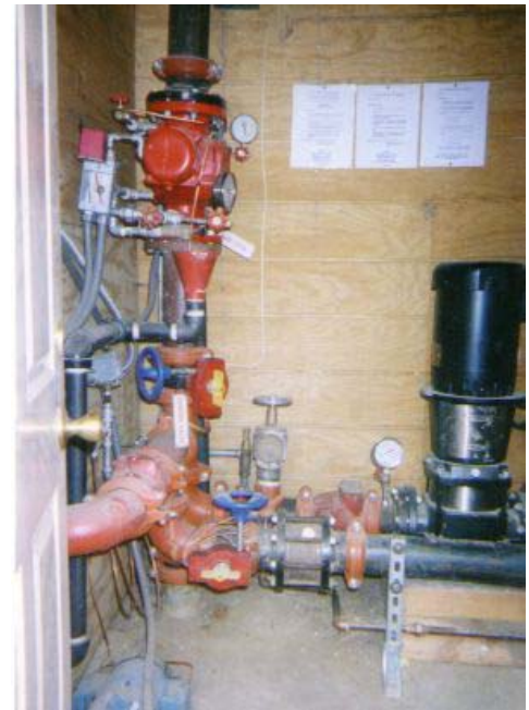
Fire Pump and Riser in Eagle Lodge
