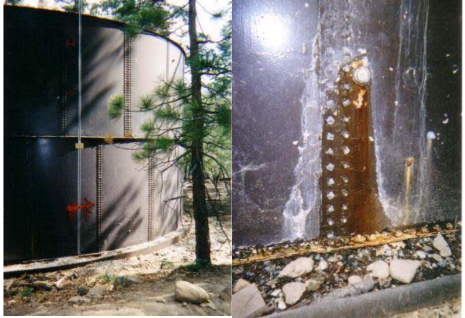
88,000 Gallon Painted Bolted Steel Water Tank Showing Leaking Plug
