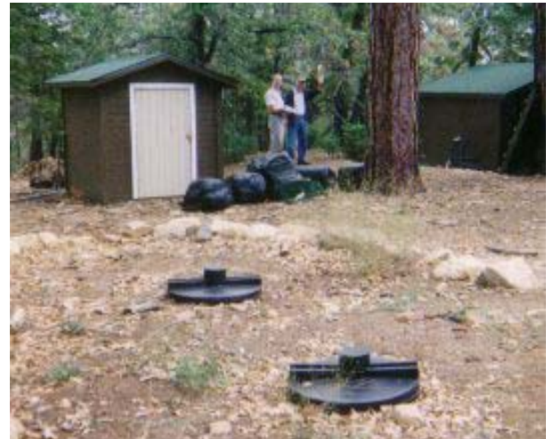
Below Ground Irrigation Storage and Shed with Booster Pump and Hydropneumatic Tank
