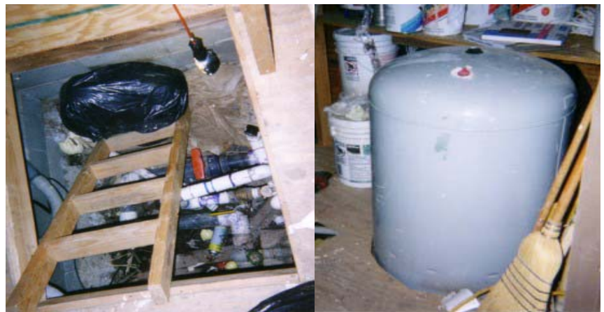
Electric Booster Pump in Vault and Hydropneumatic Tank For Potable Water System
