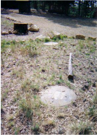
Typical Septic Tank Access Manholes
