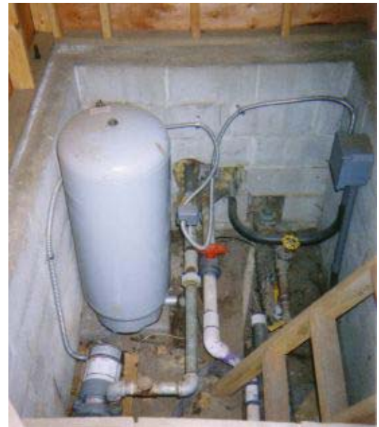
Hydropneumatic Tank and Electric Booster Pump for Irrigation Water System
