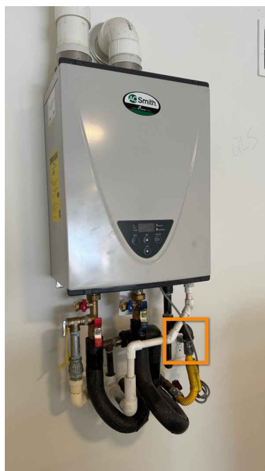
Water heater missing GFCI protection
