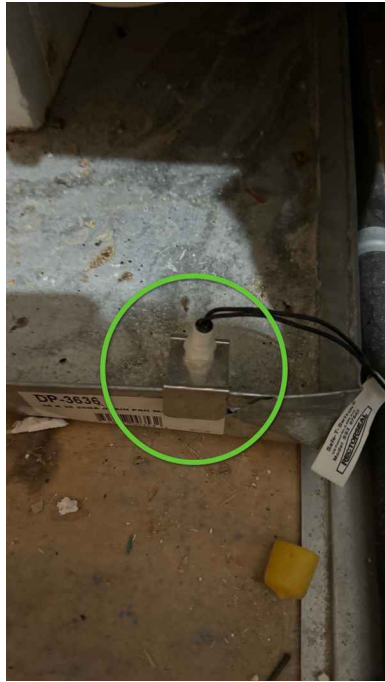
Float Switch Attic Pan
