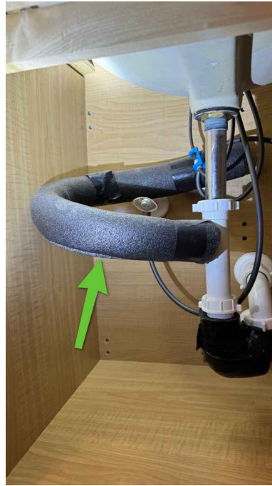
Primary Condensate Drain Primary Bathroom Sink
