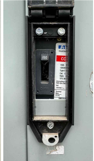
Main Shutoff Left Side Of Home
