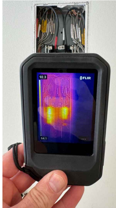
Sub Panel Garage
