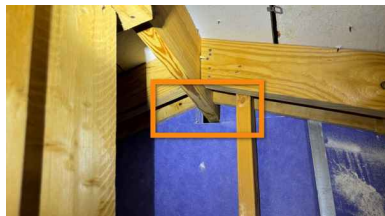
Attic Right Side Of Home. Small area should be sealed to be fully fire
