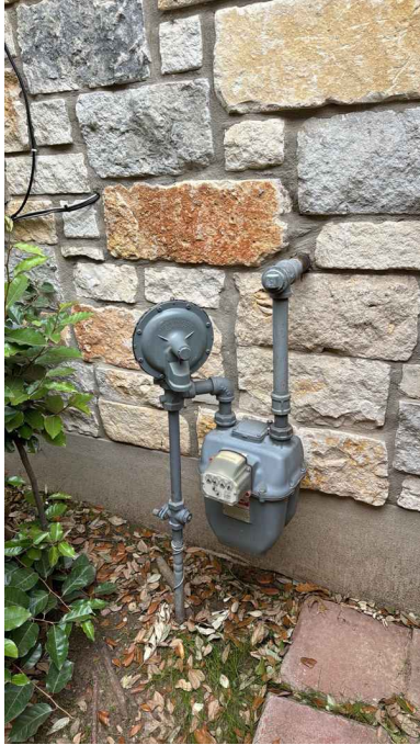
Type of Gas Distribution Piping Material: Black Iron Comments:
