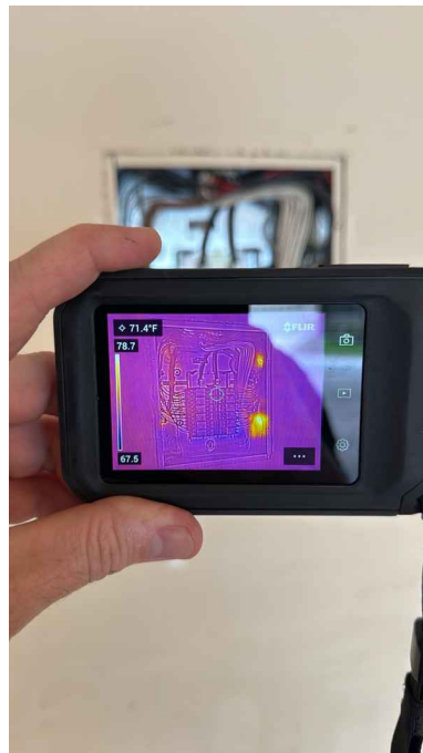
Sub Panel Garage
