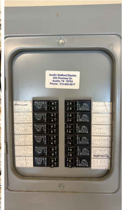
Sub Panel Garage
